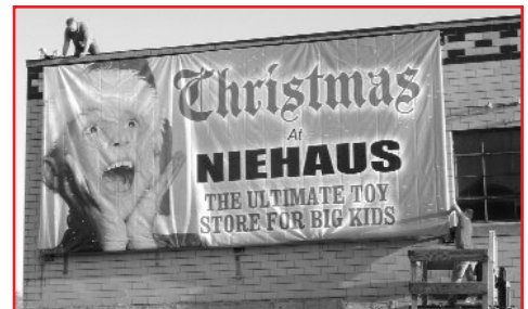
Phil, Danny and Doug work to hang the new Christmas banner on the side of the Ford Building.
