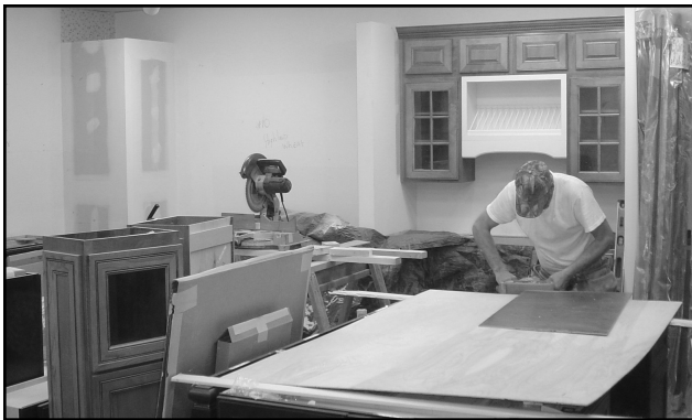
Work in progress to update and expand the showrooms at WBM in St. Louis.
